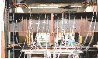
図-6 床版の圧壊
